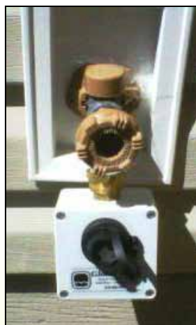
Device used for checking water pressure
